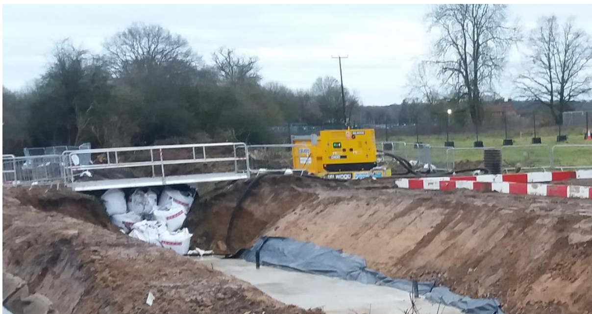
Fig 3. Above photo taken (16 January 2021) diversion of Newyears Green Bourne – concreting of river bed.
